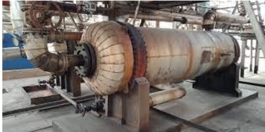
Gambar 3.1 Heat Exchanger 2 PPSDM Migas Cepu
